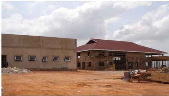
Sweden Ghana Medical Centre, under construction, in March 2010, Oncology building and reception block.
